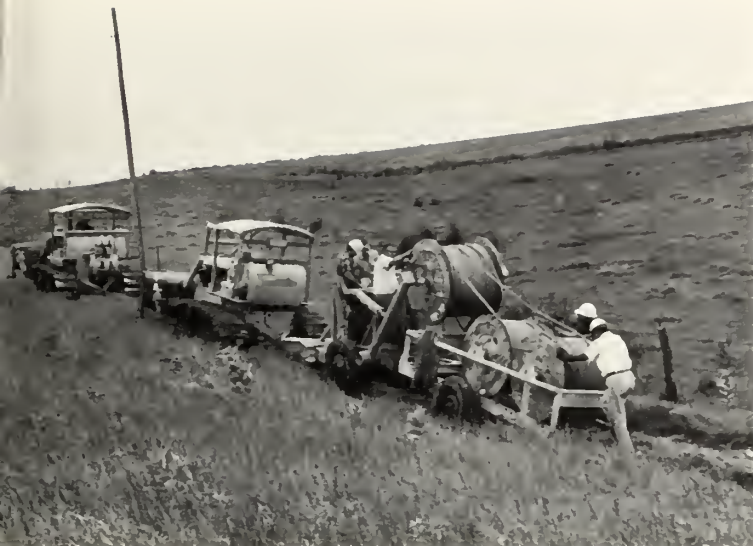
Complete undergrounding of electric distribution systems preserves the natural beauty of the countryside.
